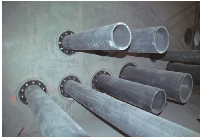
A combination of Century-Line® Sleeves and Link-Seal® Modular Seals perform a “No Leak Solution” for this pump room application.
